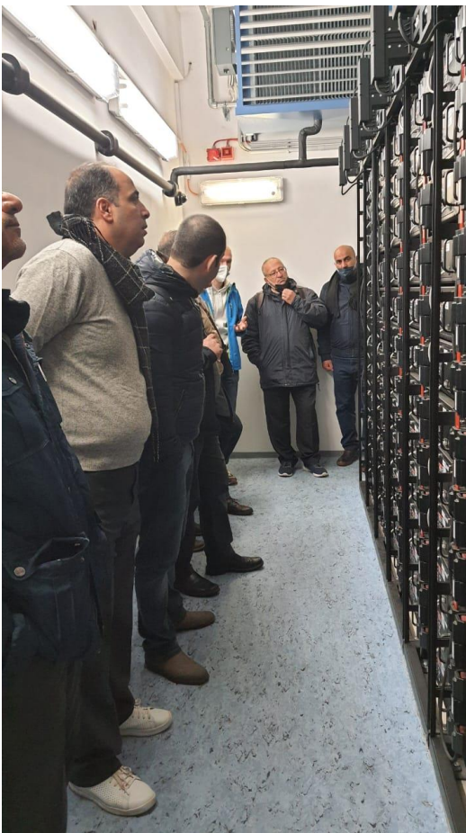
Visit of large-scale 5MWh storage:
